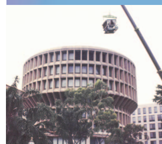
Newcastle City Council - NEW CHILLERS.
